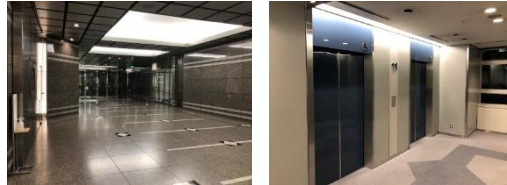
Conversion to LED lights at the entrance hall and common spaces on each floor
