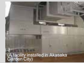
Emergency power generation facility
